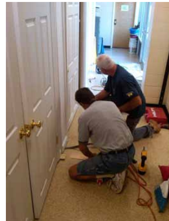
Todd and Kevin putting the finishing touches on the Cabinets. Great work guys!
